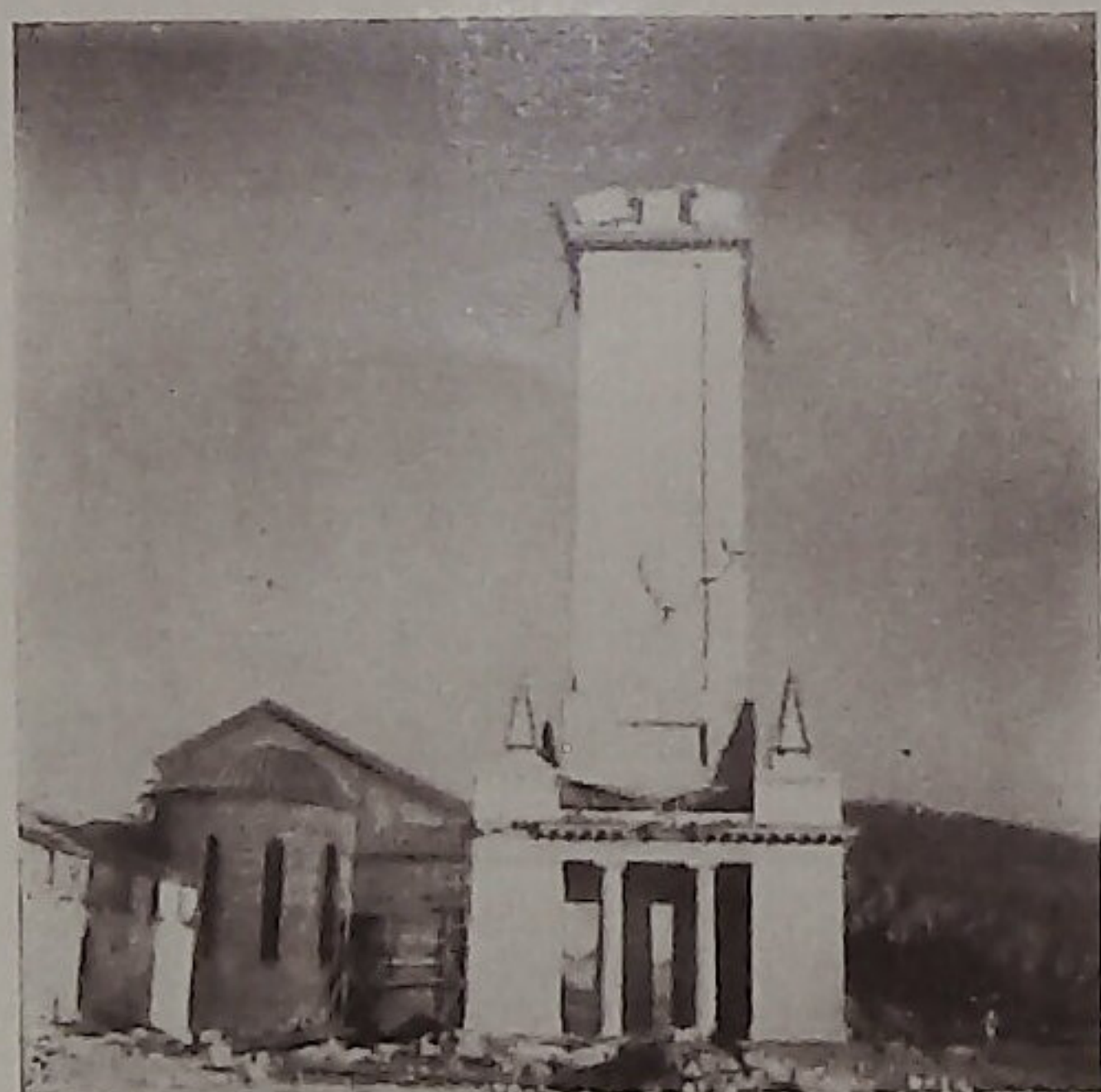
Fig. 6.—The bell tower of the Cathedral, Zante, the upper part of which collapsed and the rest badly cracked. The Church behind, designed and built to be earthquake resistant, left intact.
