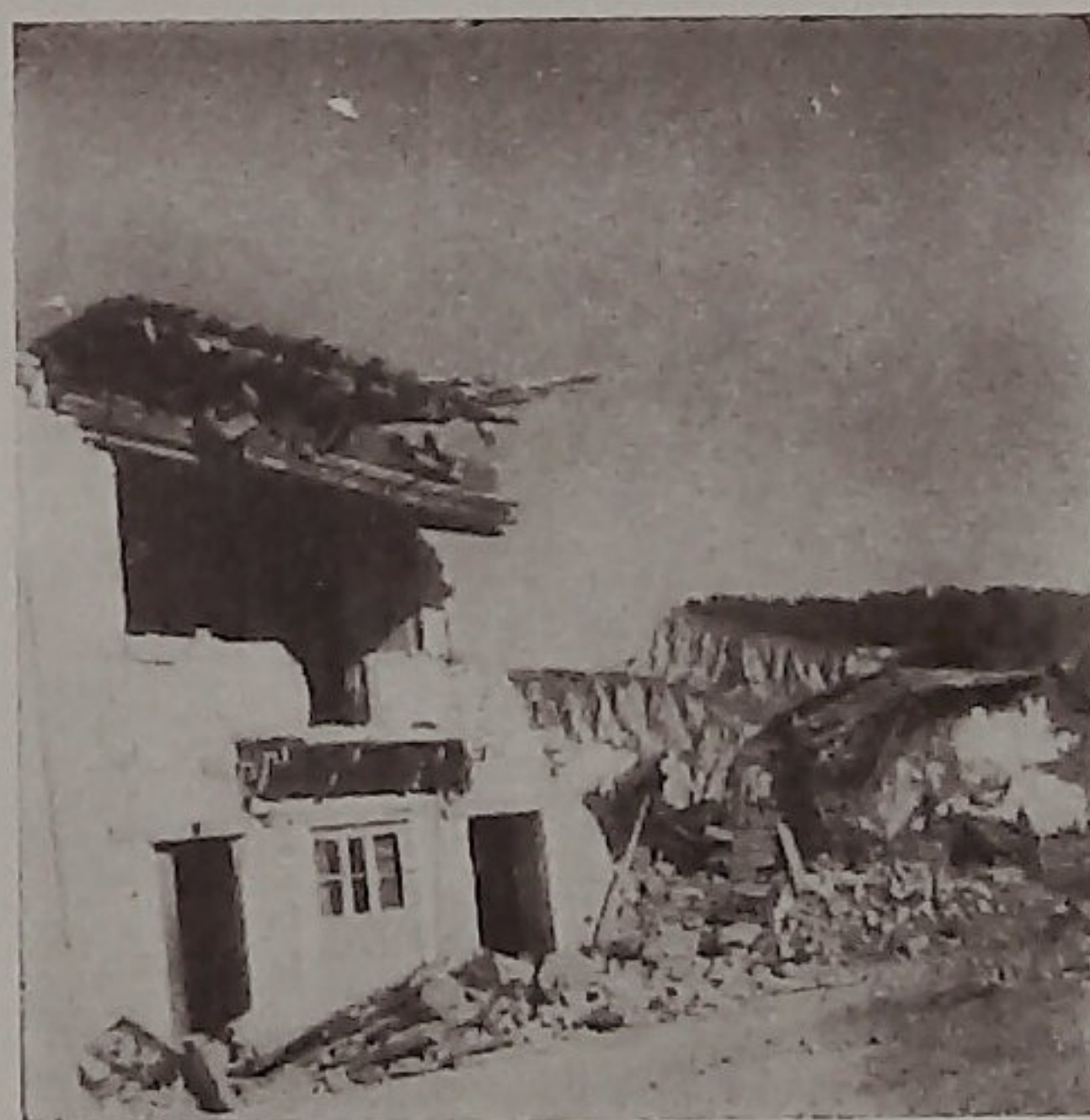
Fig. 7.—A picture of damage done to buildings of stone or brick construction in Zante.
