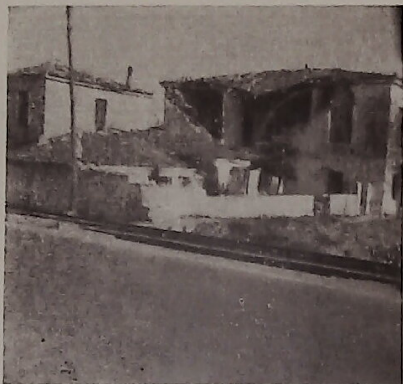
Fig. 15. — Common type of earthquake failure to old stone houses, in Agria, during the earthquakes of April 19 and 21, 1955. Note, that the new stone house on the left hand was left intact.
