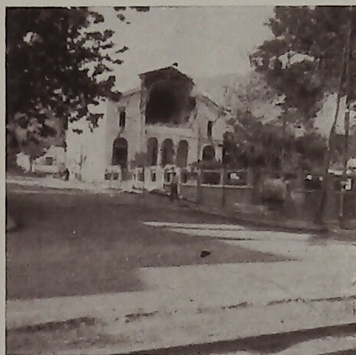
Fig. 12. — Destruction to the western side of the church, Saint George, in Agria during the earthquake of April 19, 1955.
