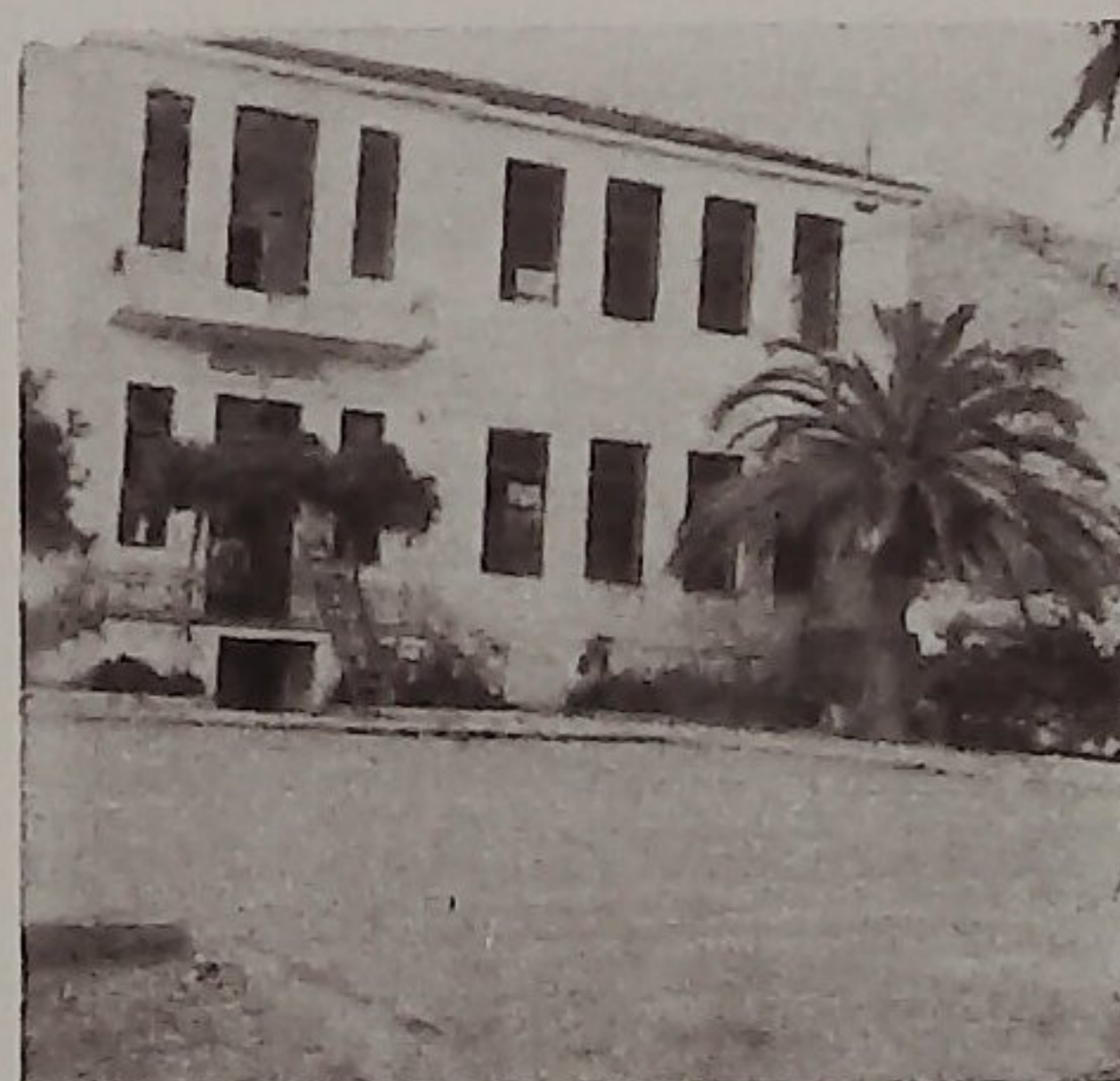
Fig. 14. — The outside of the elementary school, in Agria, after the earthquakes of April 19 and 21, 1955.
