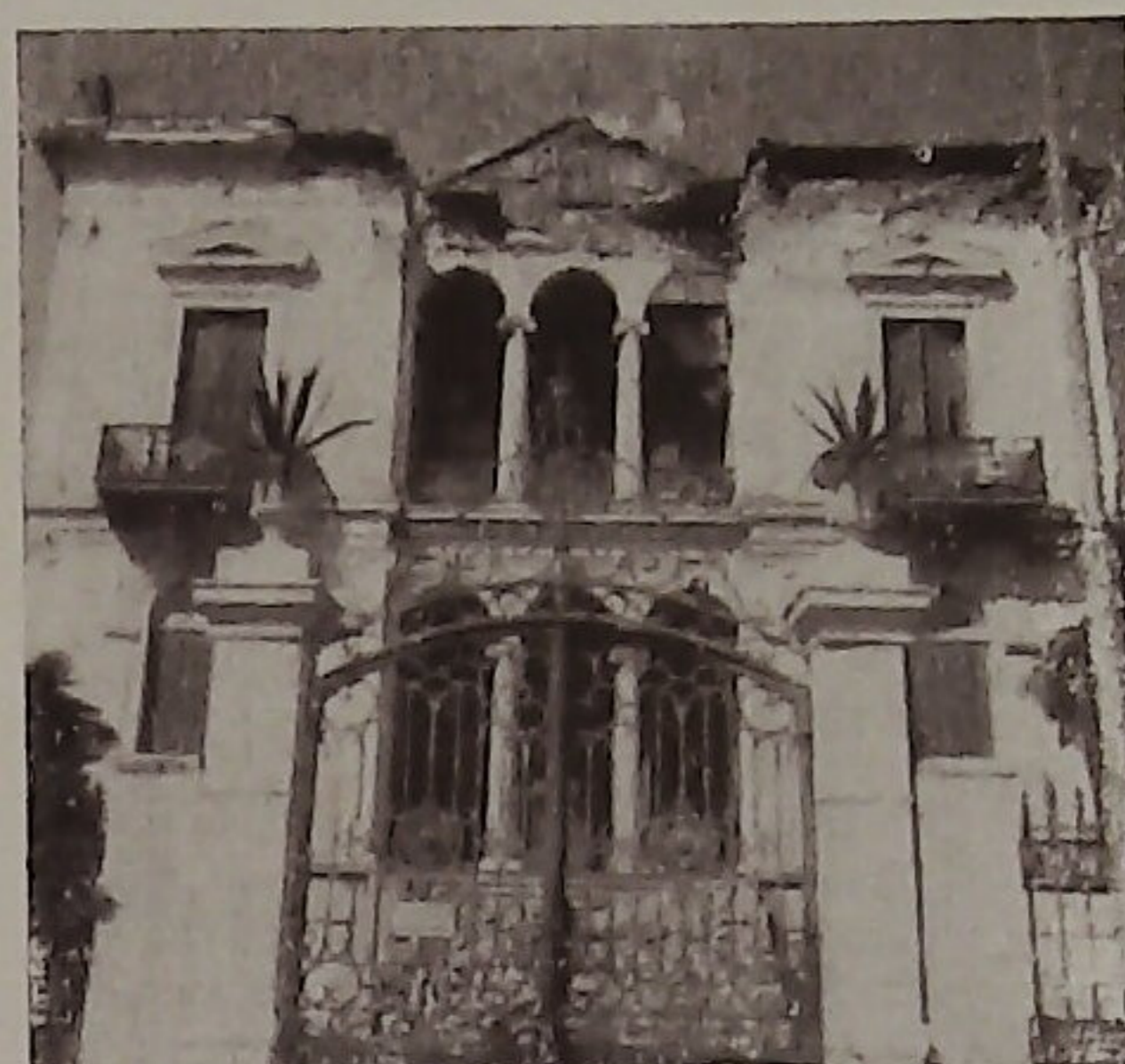
Fig. 4. — Collapse of the gable of a private clinic in the central square of Volos during the earthquake of April 19, 1955.
