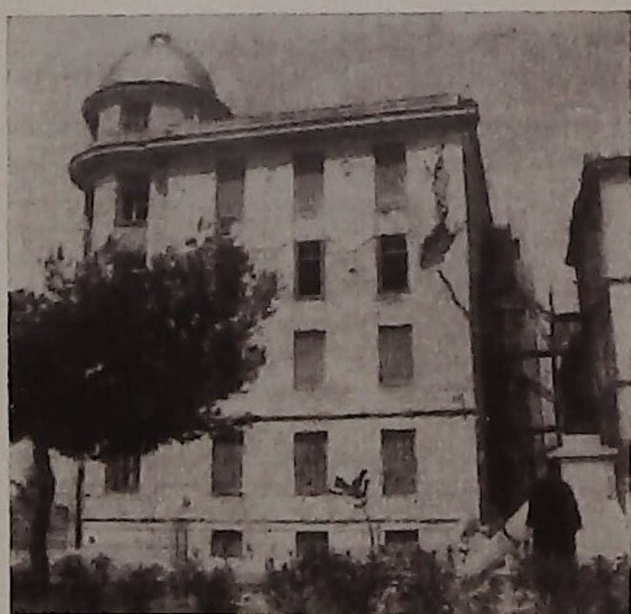
Fig. 5. — Damage to a well - built five-story building resting on man-made fill near the quay of Volos during the earthquake of April 30, 1954.
