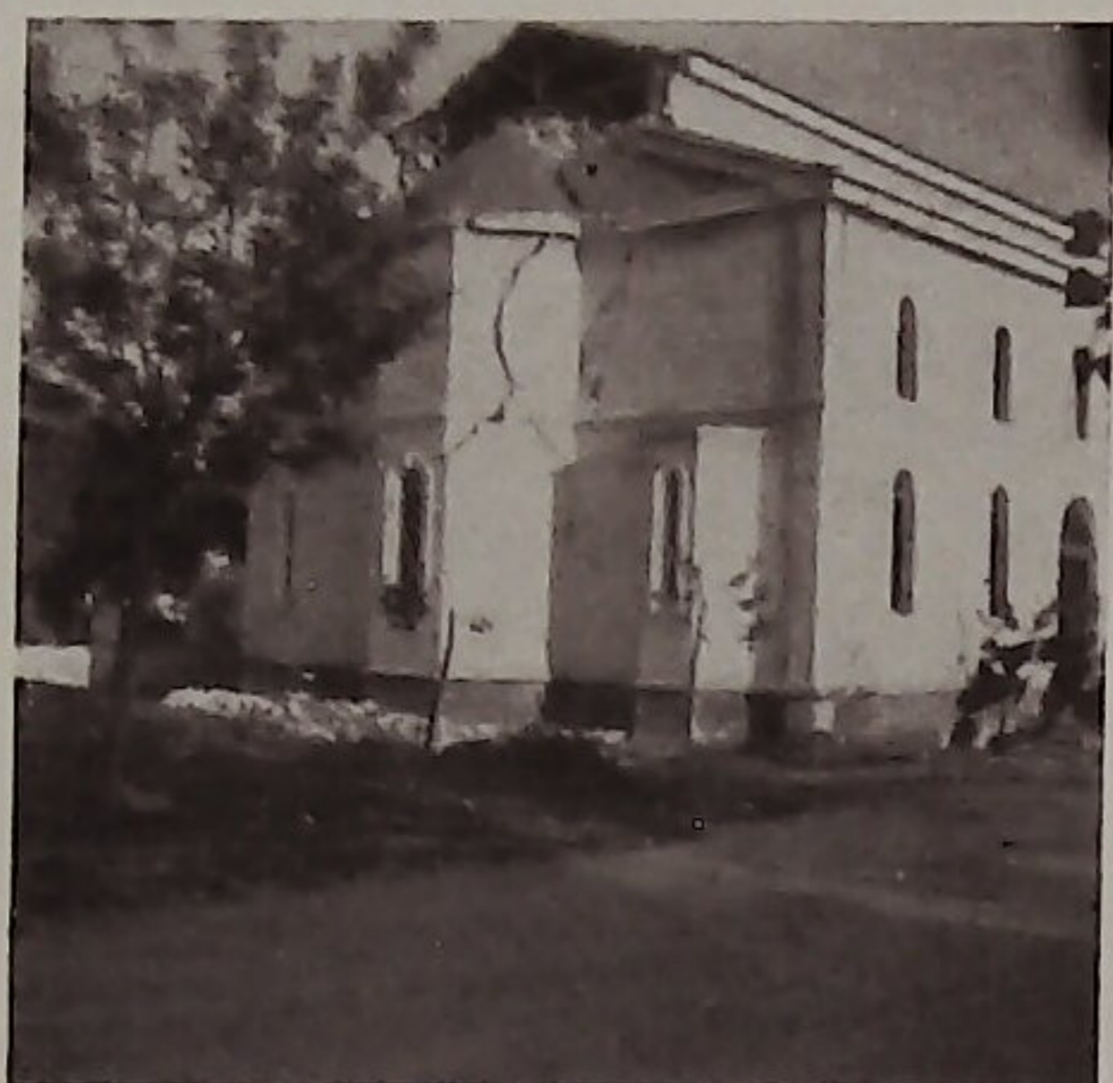
Fig. 11. — Destruction to the eastern side of the church, Saint George, in Agria during the earthquake of April 19, 1955.
