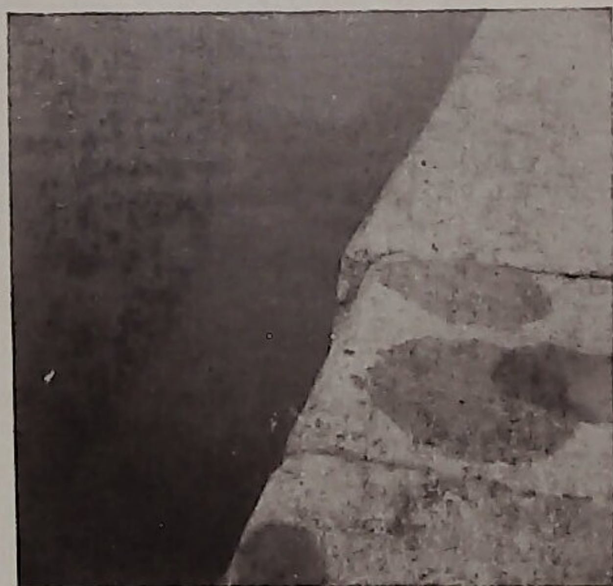
Fig. 9.—Horizontal shifting of the mole bank in the quay of Volos during the earthquake of April 19, 1955.
