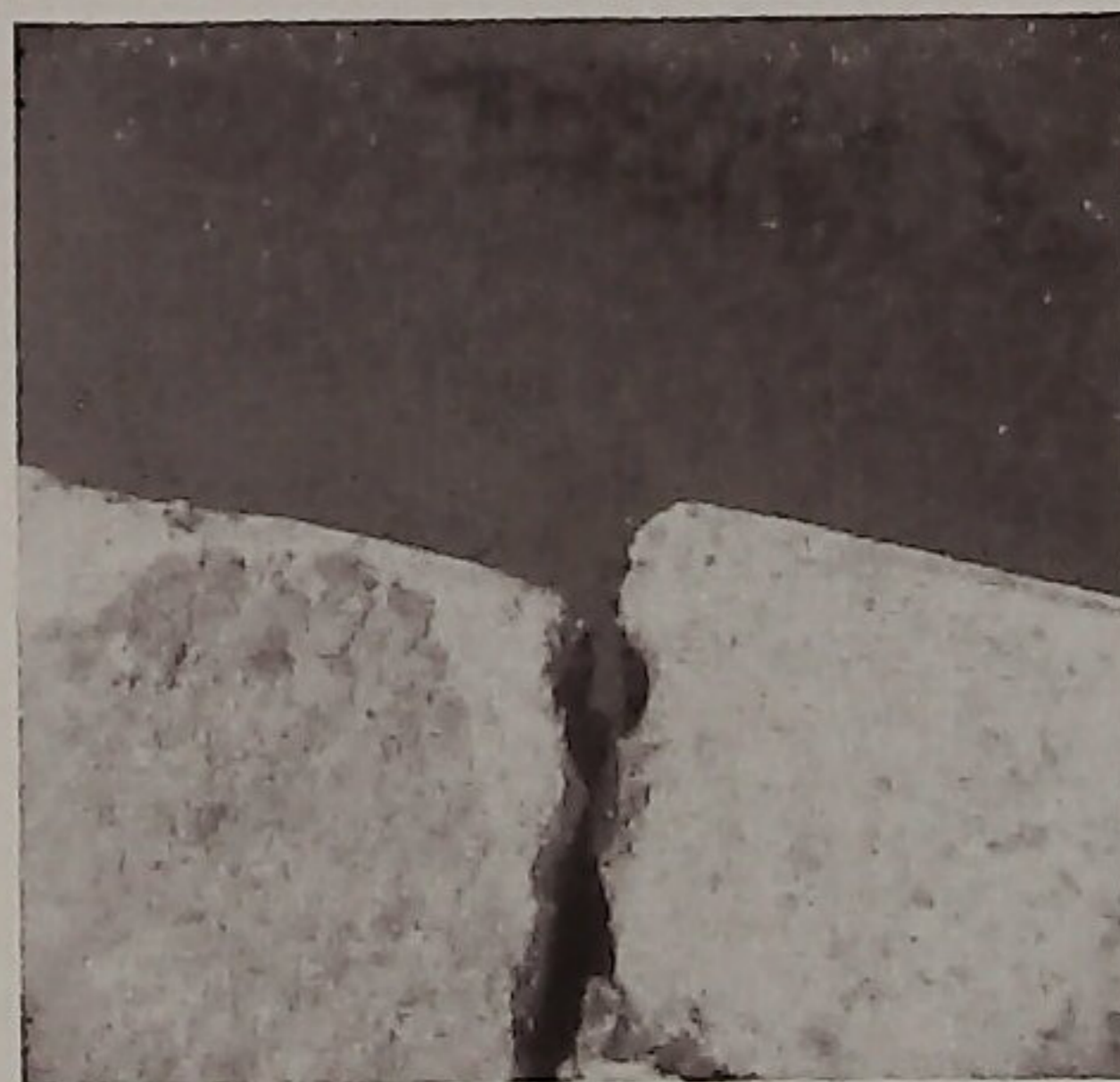
Fig. 10.—Another sight of the shifting of the mole bank during the earthquake of April 19, 1955.
