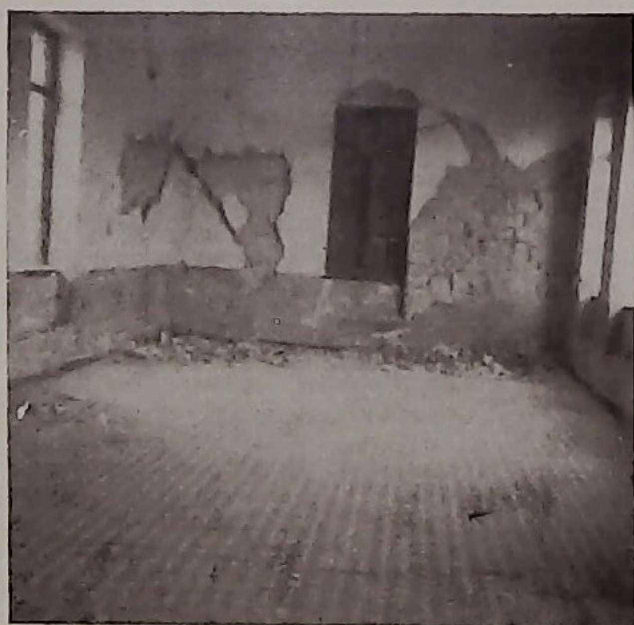
Fig. 13. — Damage to the interior of the elementary school, in Agria, during the earthquakes of April 19 and 21, 1955.
