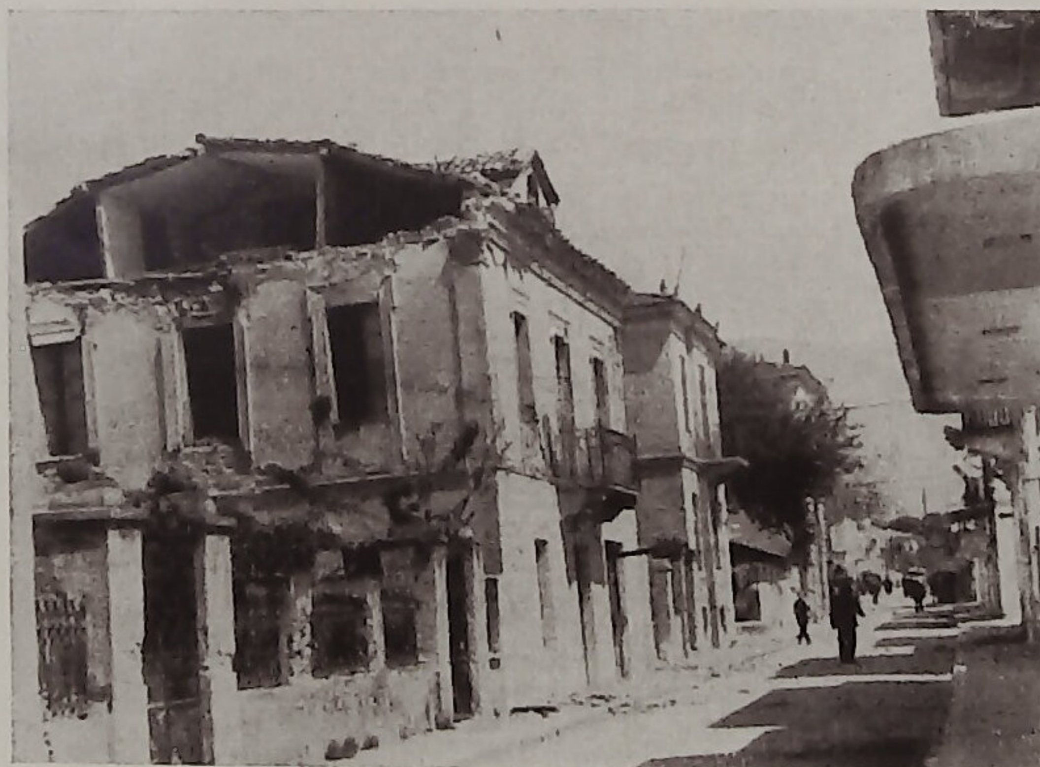
Fig. 2. — Another sight of the earthquake failure in Volos after the shocks of April 19 and 21, 1955. Note, that the second stone house on the left hand was left intact.
